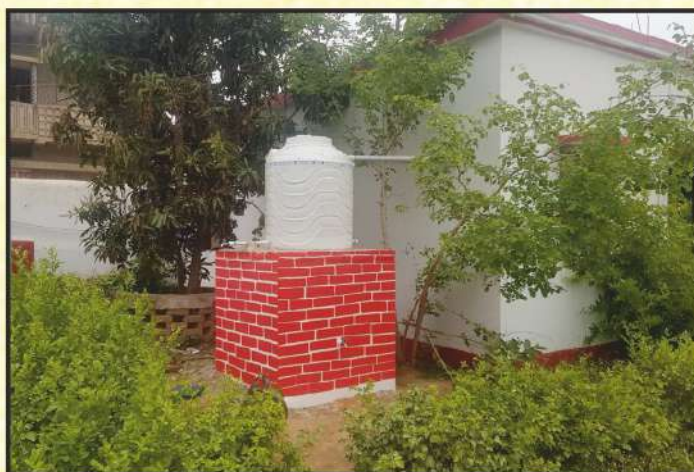
RAIN WATER HARVESTING
